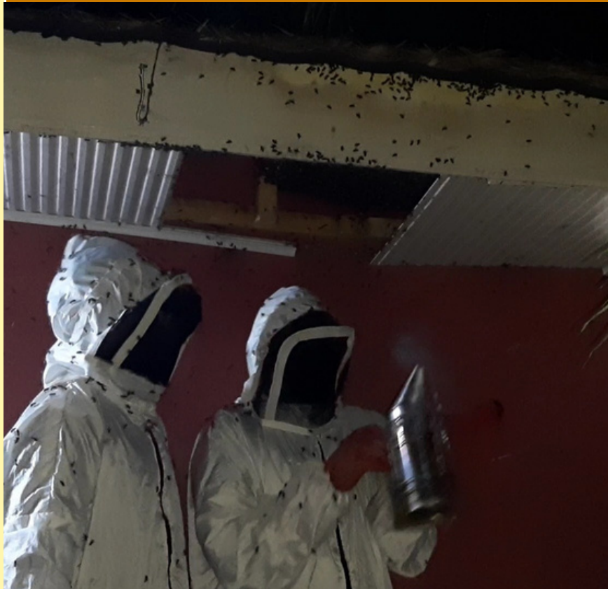
Tunza Nyuki team removing and relocating an aggressive bee colony from a House
